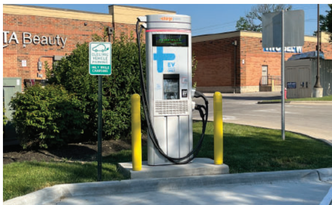
Level III EV Charger - Shoppes at Hunters Run
