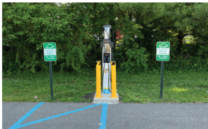
Level II EV Chargers - Olde Village parking lot
